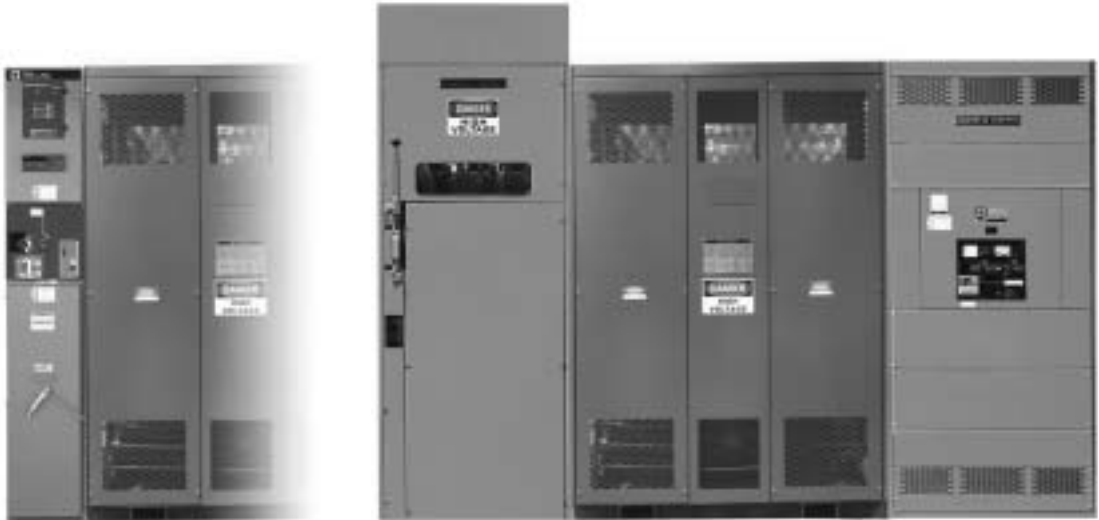
with HVL/cc Switchgear
