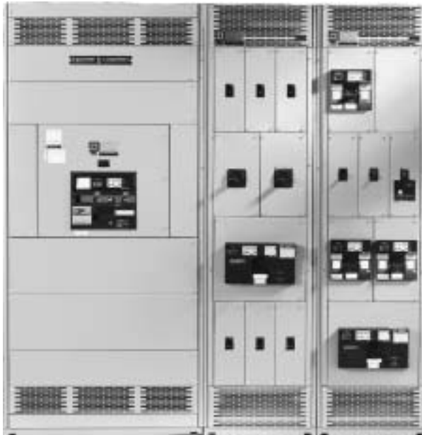
QED-3 Distribution Sections with QED Main
