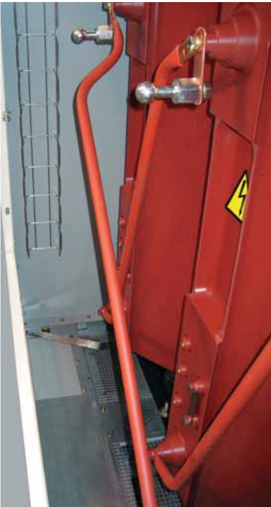
bracket for HV cables entering the bottom of the enclosure
