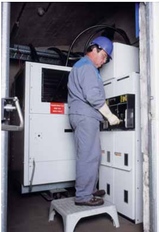
commissioning after checking
