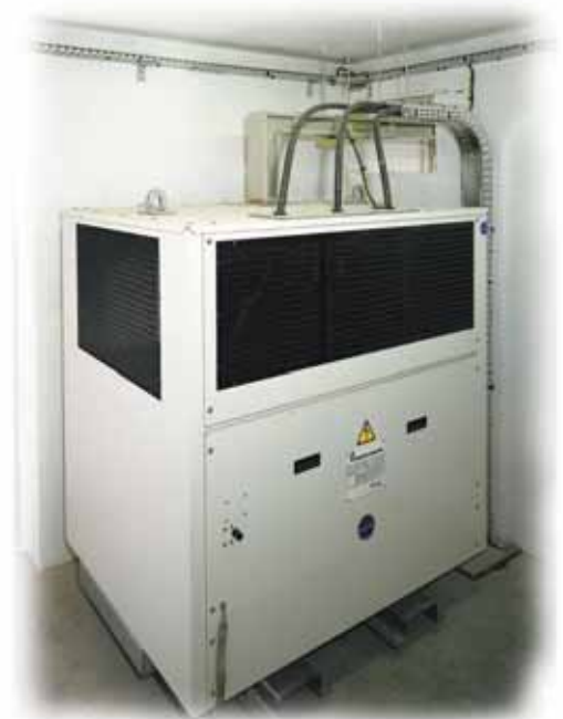
figure 4 - LV connections with PBT on enclosure
