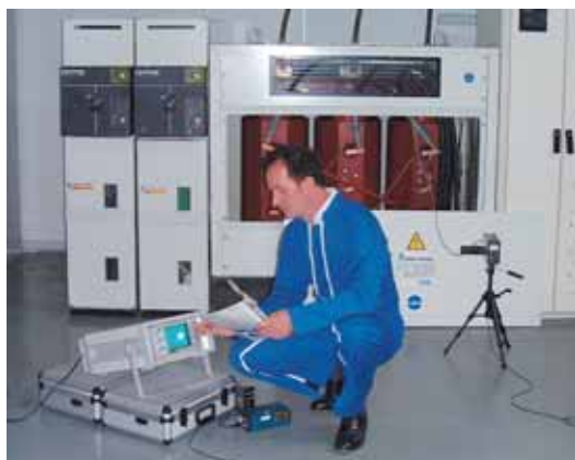
checking before commissioning
