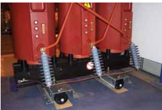
high voltage surge arresters on the lower part
