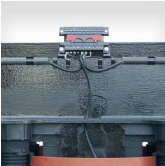
terminal block to connect sensors to the electronic converter
