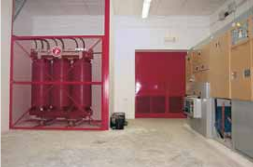
Trihal transformers (IP 00) installed on the universal exhibition from Seville, Expo 92
