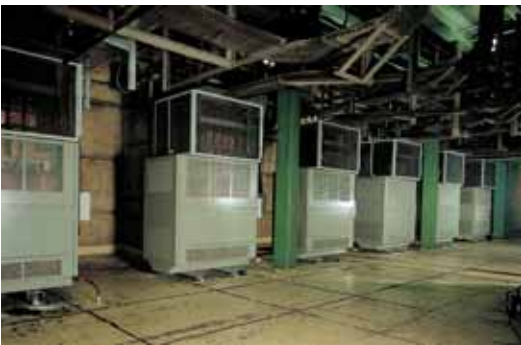
Trihal transformers with IP 31 metal enclosure installed in a steel works
